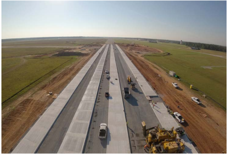
U.S. Air Force Lt. Col. Alvin McConkey, director of inspections for the 169th Fighter Wing's Inspector General's office, uses his drone to acquire photo and video imagery of the runway construction at McEntire Joint National Guard Base, South Carolina, September 21, 2022. McConkey is a licensed drone pilot and is assisting public affairs in acquiring arial footage of the runway construction. (U.S. Air National Guard courtesy photo by Lt. Col. Alvin McConkey, 169th Fighter Wing)
